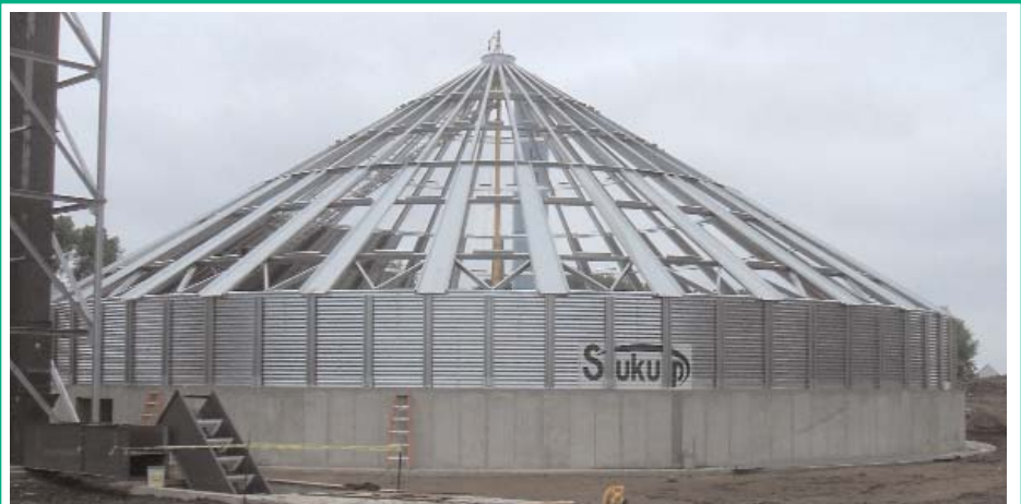
Throughout the past month several project milestones have been met. Within the last few days the Thor Project has progressed into the "bin-jacking phase". This photo shows one of two completed bin roofs along with the first two rings. Upon completion of the "bin-jacking phase" we will transition into the "millwright phase".
